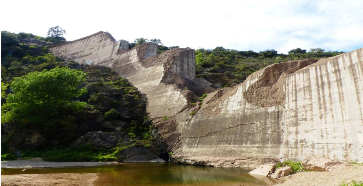
Remains of the dam
