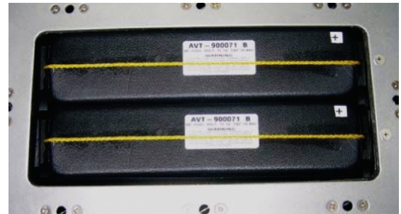
Cover removed, exposing 2 Lithium Ion batteries
